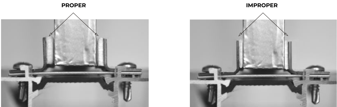
Photo 14. Proper mounting (felt washer, not deformed) and improper mounting (lack of clearance caused by non-parallel screwing of steel angle bar or by use of inappropriate angle bar)
